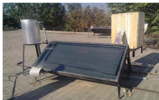
Figure 9: Solar collector with water warming tank (Hanif et al., 2016).
